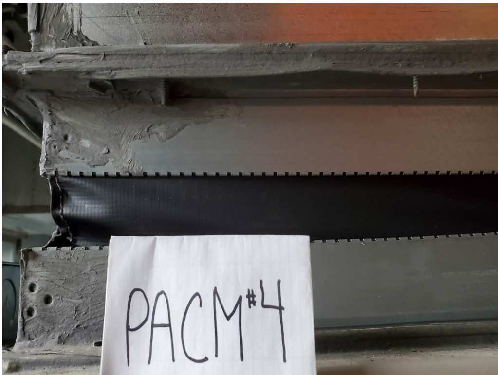
PACM #4 – Vibration dampening Cloth
